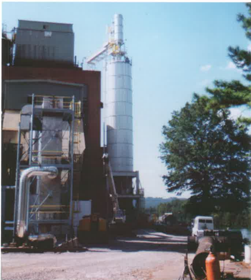
The silo supplier designed this 500-ton-capacity silo to structurally support the vacuum collector and other equipment mounted on its top.
