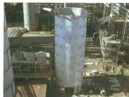
This bolted steel silo is being erected one ring at a time.
